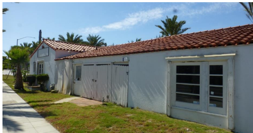
The once-prominent Woodruff Tract Office now sits vacant and in need of repair.
